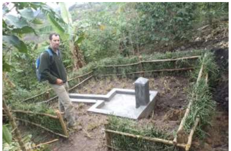
Constructed tapstand at Ndere water supply being appreciated by Ben Thorne from UK
