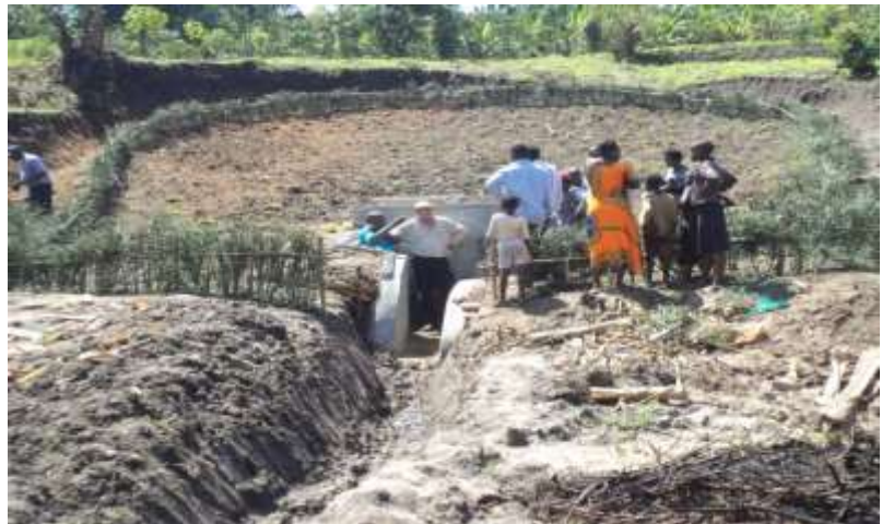
Supervision of the finished construction of Bwambara spring by WATSAN Staff together with the visiting of Andrew Maclean
