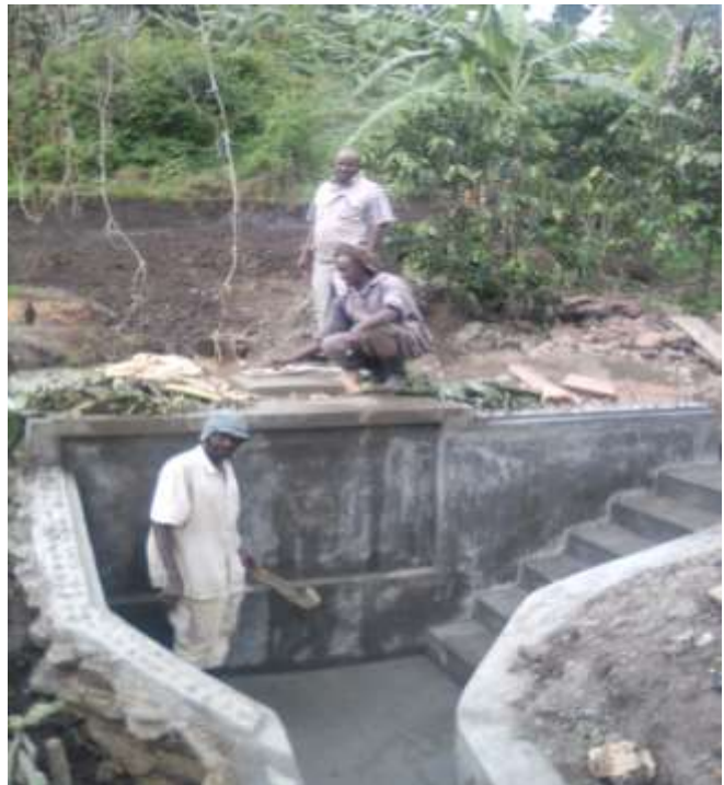
Supervision of Mabanga spring construction by Coordinator & his team slightly before it was finished in September, 2018
